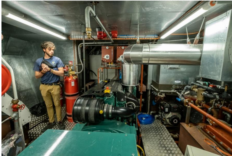
Fig 3.8: The ship is electrically powered and recharges at night, at the quayside.
