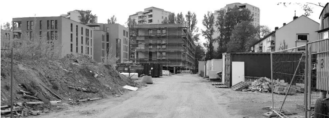
Figure 3.4: Traffic route for construction vehicles past office and recreation containers (Photographed in Essen, Germany, 2021)
