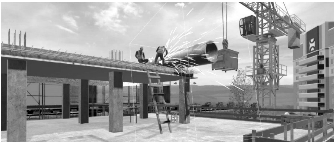
Figure 5.11: Hazard area, two workers with an angle grinder
