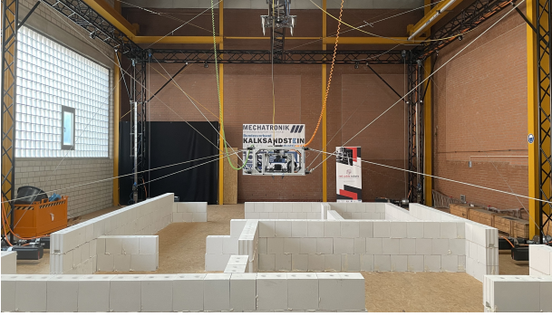
(a) CARLO prototype in Duisburg for automated masonry construction using calcium silicate units and mortar.
