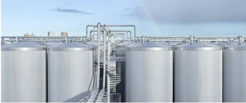
Figure 7.8: An example of tank systems 1
