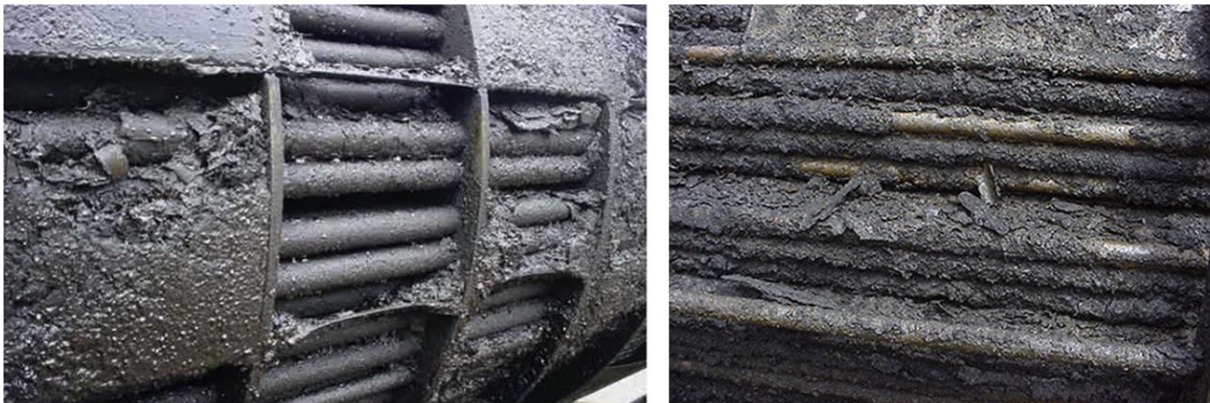
Figure 1-2: Fouling on the shell-side of refinery heat exchangers.
