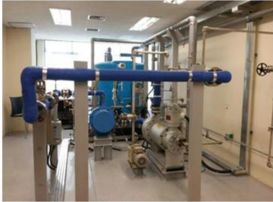
Figure 6. General view of SCO 2 PE
