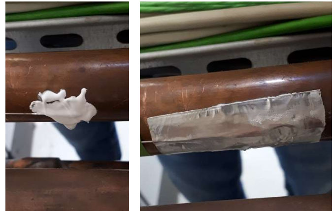
Figure 3: Installation of Ø 0.75 mm thermocouple at the surface of the pipe with a layer of thermal paste (right) and covered with aluminium tape (left).
