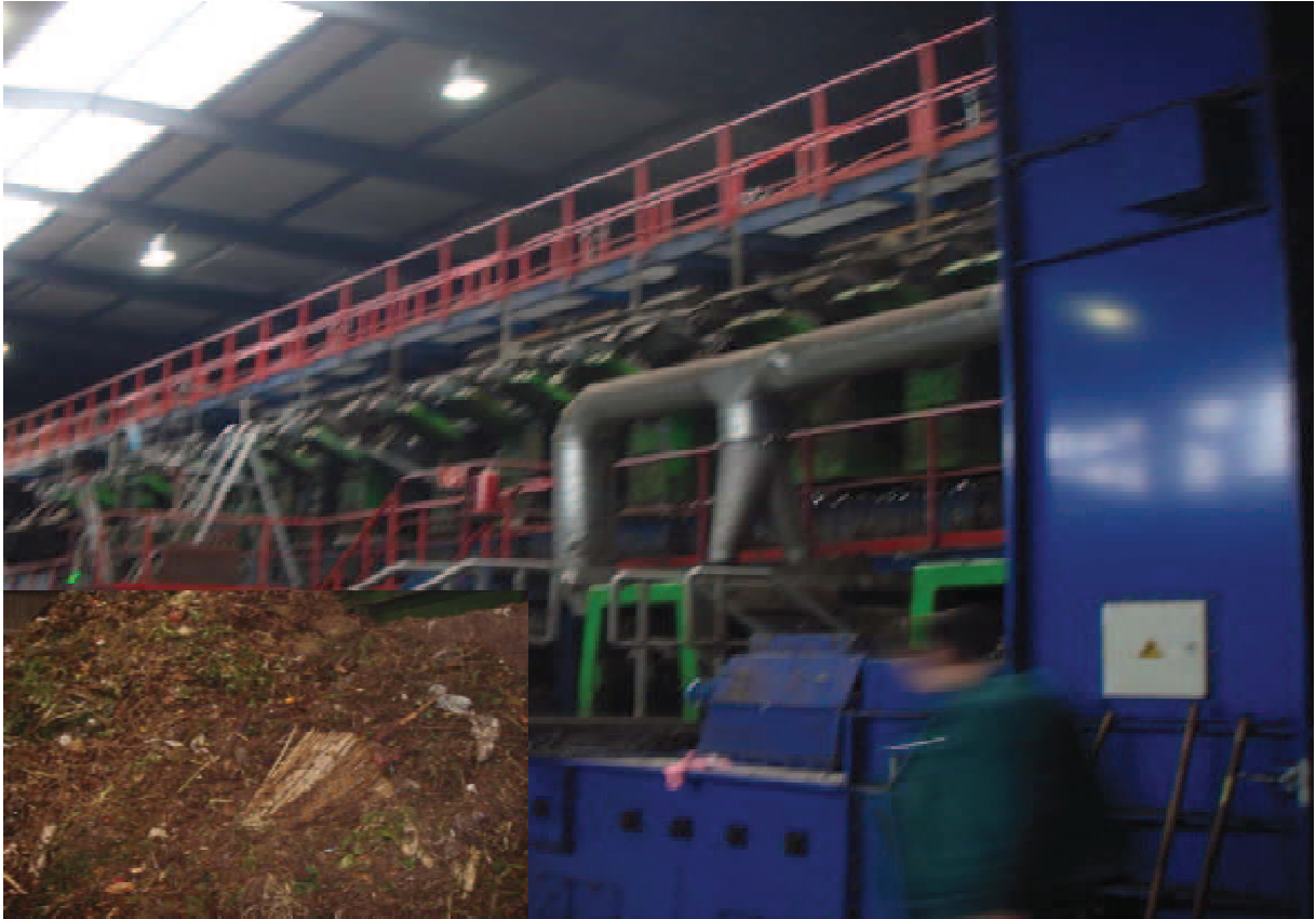
Figure 2-2: Biological Waste Plant for the Methanisation and Composting.
